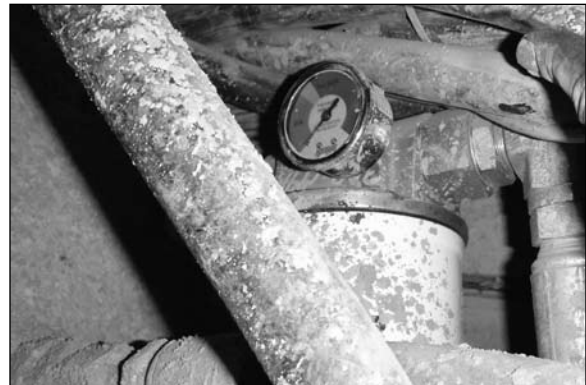
Filter Indicator On Front Hydraulic Car #6
