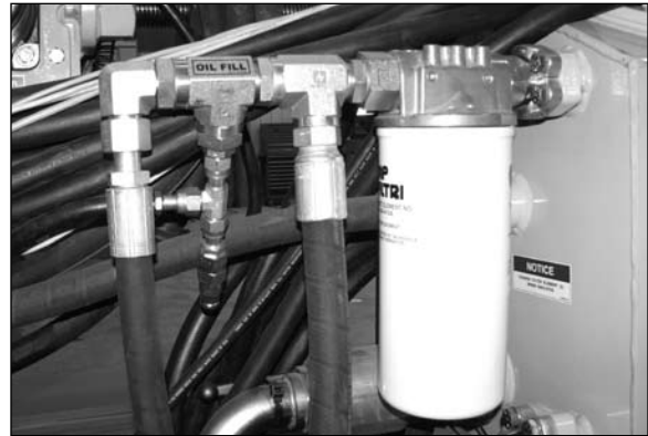
Front Hydraulic Car #6 Hydraulic Fill & Reservoir
