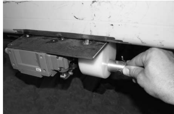
Pushing In Spool Of Belt Stop Control On Incline Belt Car 1
