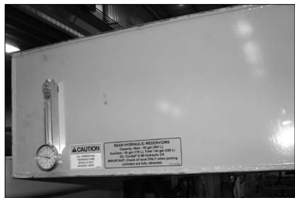
Rear Hydraulic Car #7 Auxiliary Reservoir
