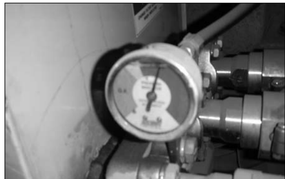
Filter Indicator On Rear Hydraulic Car #7
